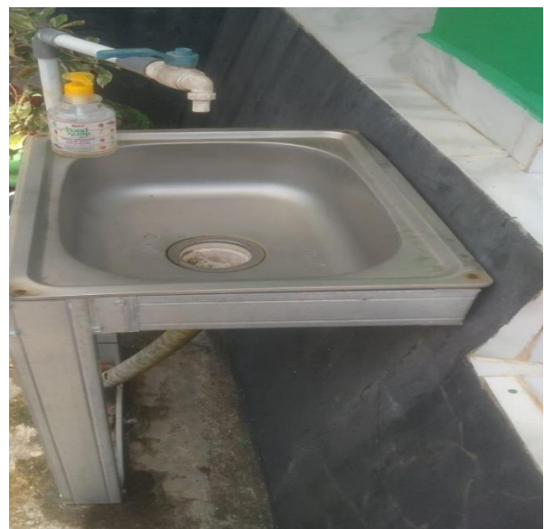
Figure 1. Hand Washing Facilities
