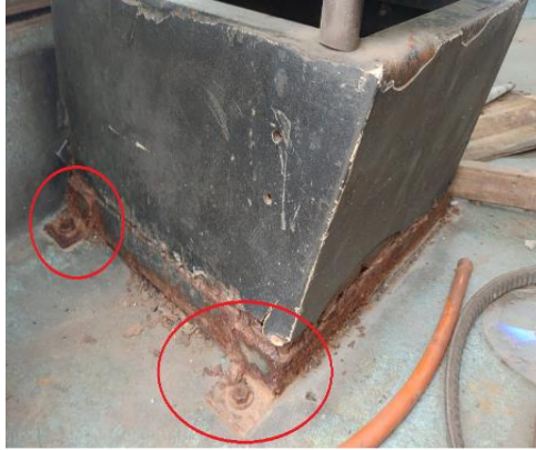
Figure 6. The actual condition of the support bolt hole after years of use
