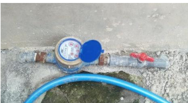
Fig. 8 Glagaharjo residents' water meter
