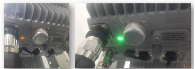
Figure 18. Hardware problem could be checked from the alarms status, check as well the transmission alarm (source: parallel wireless)
