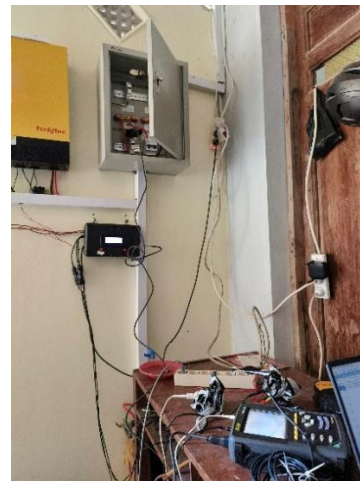
Fig. 15. Power Quality Testing
