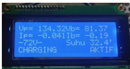
Fig. 22 Charging Battery Gesits 72V
