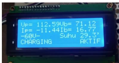
Fig. 18 Charging Battery Volta 60V
