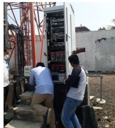
Fig. 2. Field measurement of BTS Power Radiation
