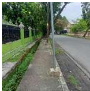
(a) No tactile paving
