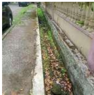
(b) No barrier between the sidewalk and the drainage system
