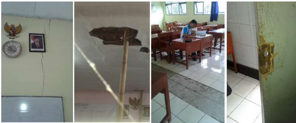
Figure 3.2. Damage of SMP Negeri 4 Salatiga
