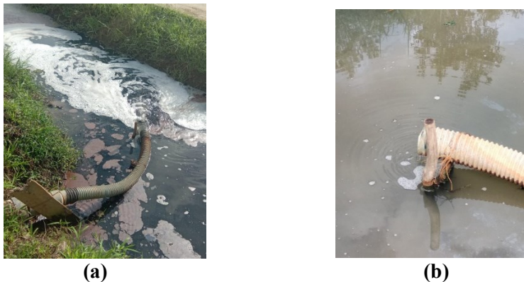
Figure 5. DWWT outlet (a) when the pump machine is operating (b) the pump machine is not operating
