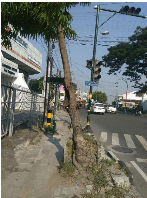
Figure 2. The damages of trees' roots (Researchers' documentation, 2018)
