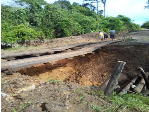
Figure 5. Landslide on the Road.
