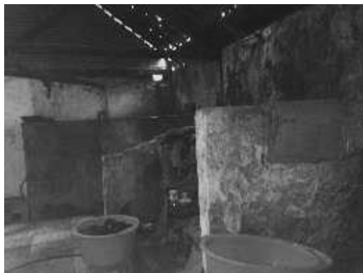
Figure 10. The Bathroom Condition
