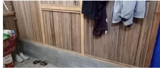
Figure 17. Good condition of the second model after 2 years of installation (interior view)
