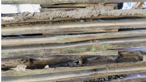
Figure 16. Bamboo damaged by termites
