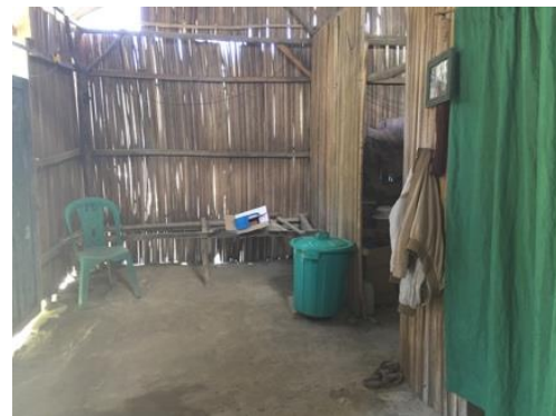
Figure 2. Air gaps in the bebak wall Source: Author, 2017.
