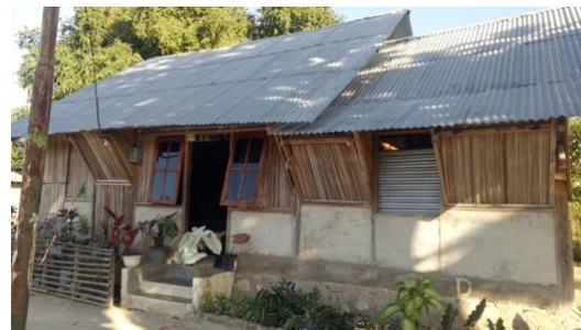
Figure 18. Good condition of the second model after 2 years of installation (exterior view)
