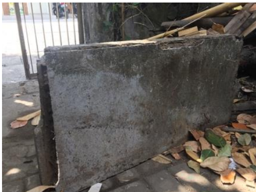
Figure 14. Moldy plaster on the exterior of the first model after 2 years
