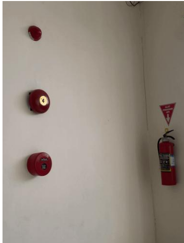
Figure 5. Fire Alarm and Fire Extinguishers in Library of UII
