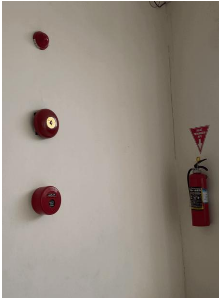
Figure 5. Fire Alarm and Fire Extinguishers in Library of UII
